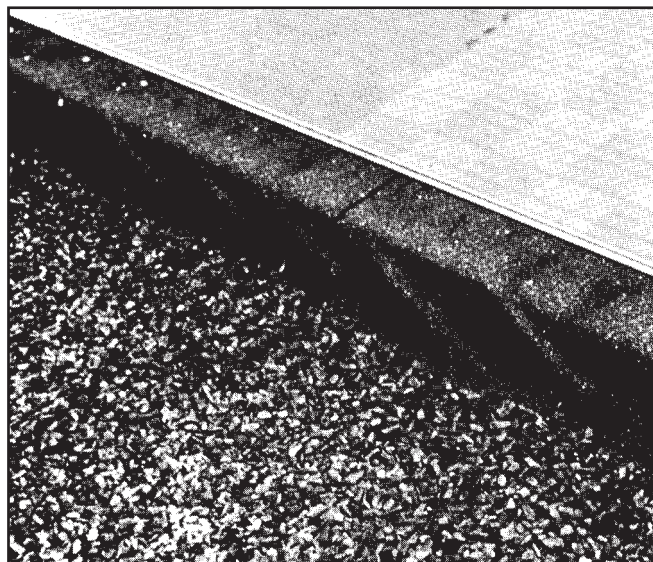
A sure sign of differential movement between the roof structure and the wall
